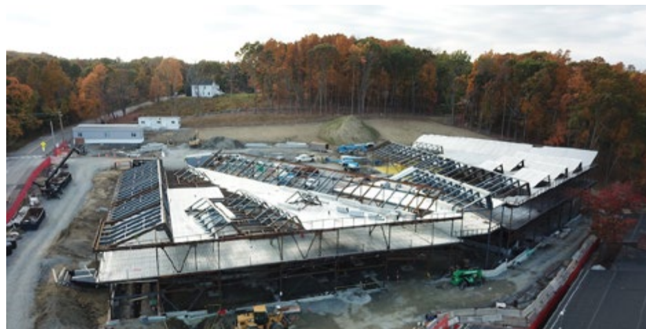
Aerial view of the Fales Elementary School building site / Photo courtesy of Gilbane Building Company
